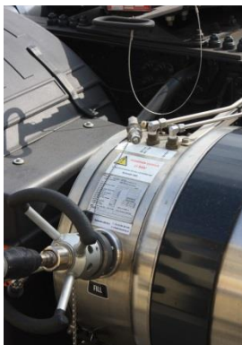
Connection of supply hose to the tank.
