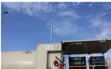
Supply installation blow-off pipe.
