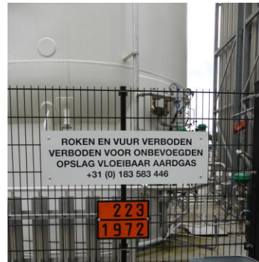
Recognisability of LNG & contact details of operator in the vicinity of the storage tank.
