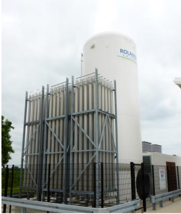
Storage tank with heat exchanger.
