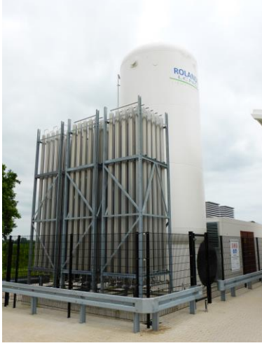
Storage tank with heat exchanger
